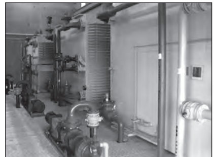
ECO-THERM® Class A Sludge Pasteurization
